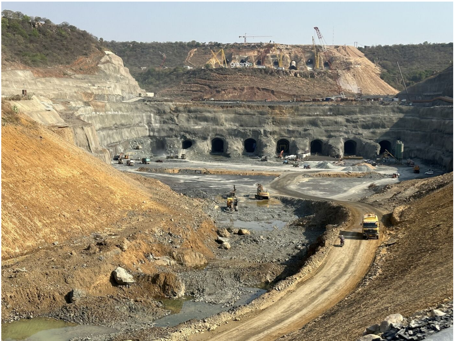
Greenko's pumped-storage facility. Photographer: Andy Mukherjee/Bloomberg
